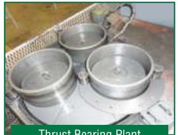
Thrust Bearing Plant
